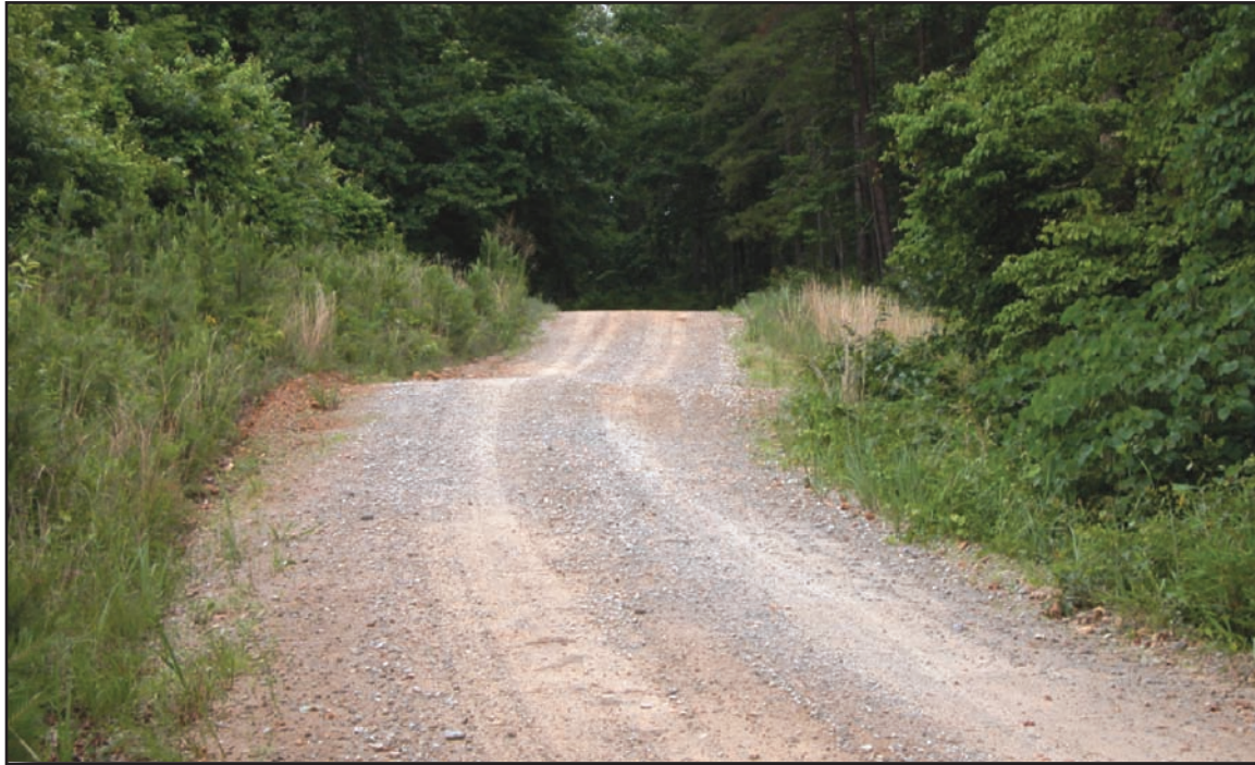
Figure 15—Maintenance level 3 single-lane road with a gravel surface, no shoulders, and a cross-drain dip. Drainage facilities, such as drain dips, should be maintained so they are functional to prevent unacceptable environmental and resource damage and to provide travel by prudent drivers in standard passenger cars. Surface roughness is acceptable if travel by prudent drivers in standard passenger cars is provided. Curves and other hazards should be marked with warning signs if advised by a documented engineering judgment or engineering study.
