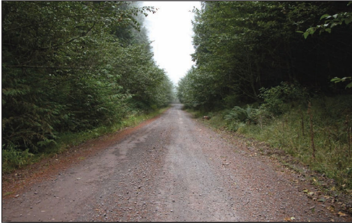
Figure 14—Maintenance level 3 single-lane road with a gravel surface and gravel shoulders. Surface roughness is acceptable if travel by prudent drivers in standard passenger cars is provided. Vegetation up to the road edge is acceptable if it does not interfere with adequate sight distance needed for a maintenance level 3 road. Brushing may be necessary on this road to provide adequate sight distance. The base course and surfacing should be replaced as needed to protect the resource.
