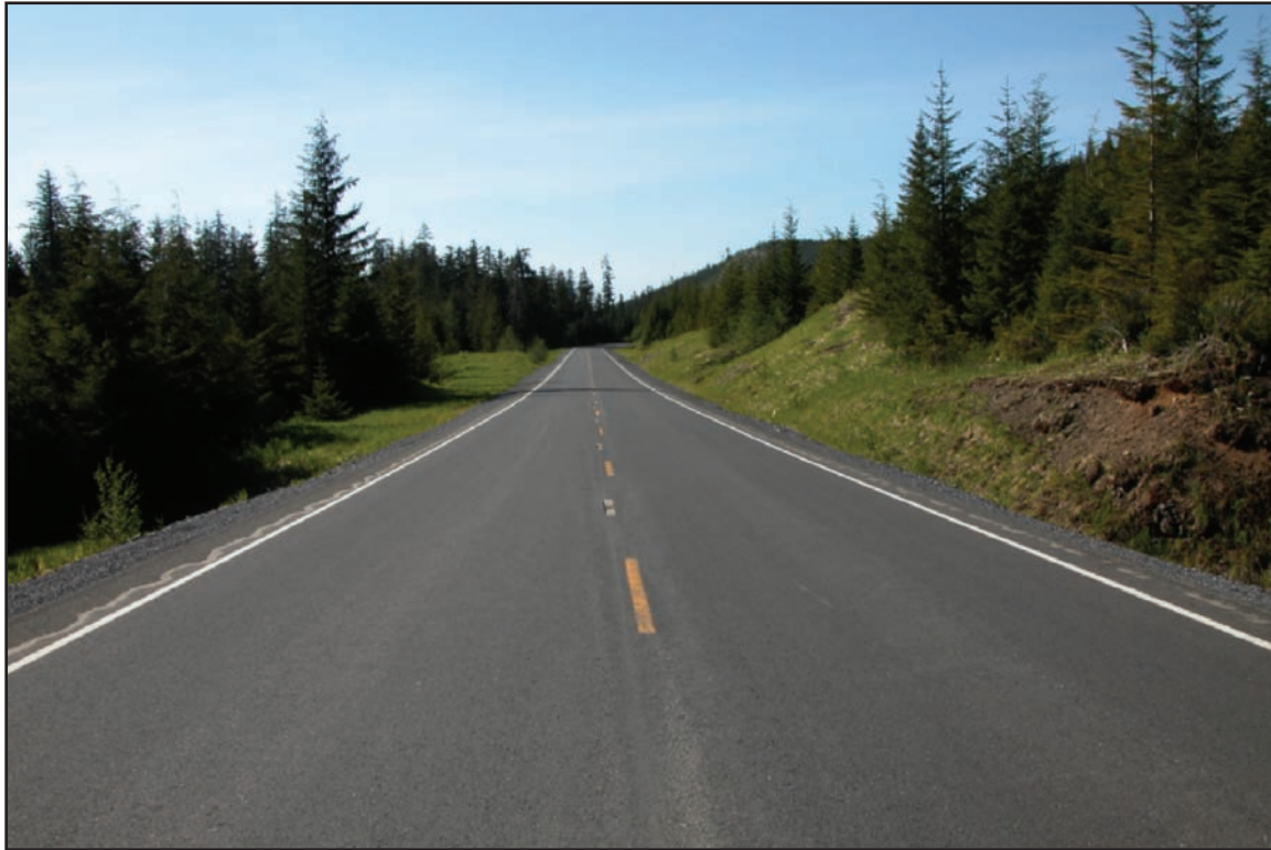
Figure 1—Maintenance level 5 double-lane road with centerlines and edge markings, a hot-mix asphalt surface, and asphalt- and rock-stabilized shoulders. If centerline markings are placed on a road, the no-passing zone markings also shall be placed as determined by an engineering study.
