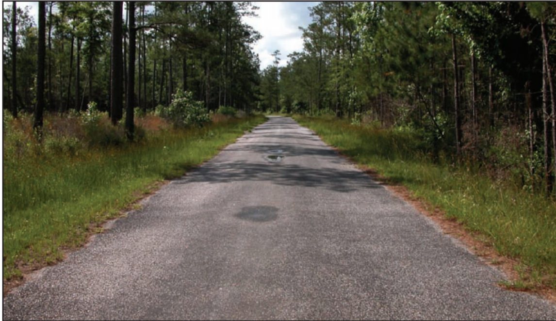
Figure 10—Maintenance level 4 single-lane road with a chip-seal surface and ditches. Potholes and depressions should be monitored and repaired before they adversely affect the user's comfort and/or convenience expected on a maintenance level 4 road. The ditches in this photo are beginning to become overgrown with vegetation, and they should be maintained properly to facilitate drainage. The road is free of litter, and the maintenance of the roadside vegetation provides adequate sight distance. Curves and other hazards should be marked with warning signs if advised by a documented engineering judgment or engineering study.
