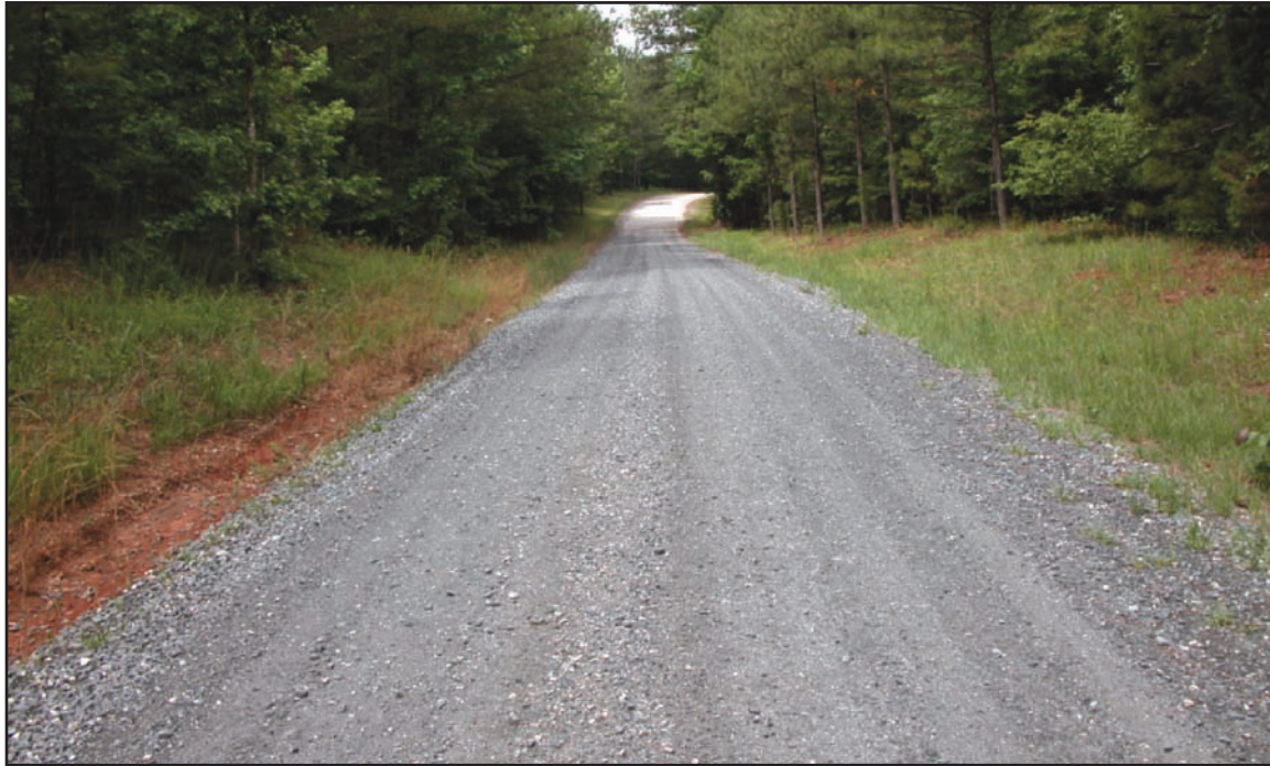
Figure 9—Maintenance level 4 single-lane road with a gravel surface and gravel shoulders. Maintain a proper crown, repair potholes, and remove washboarding to facilitate drainage and to maintain a moderate degree of user comfort and convenience at moderate travel speeds. Maintain ditches to facilitate drainage. The road is free of litter and the maintenance of the roadside vegetation provides adequate sight distance. Curves and other hazards should be marked with warning signs if advised by a documented engineering judgment or engineering study.
