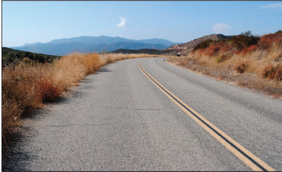
Figure 3—Maintenance level 5 double-lane road with an asphalt surface and grass on the shoulders. Speed limits may be posted as necessary with a Code of Federal Regulations (CFR) order after completion of an engineering study. Grass on shoulders is acceptable and helps with stabilization. Pavement cracking should be monitored so it can be repaired before it has a negative effect on the high level of user comfort and convenience expected on a maintenance level 5 road. Edge markings are not required on a paved road. Ditches are kept clean to facilitate drainage.
