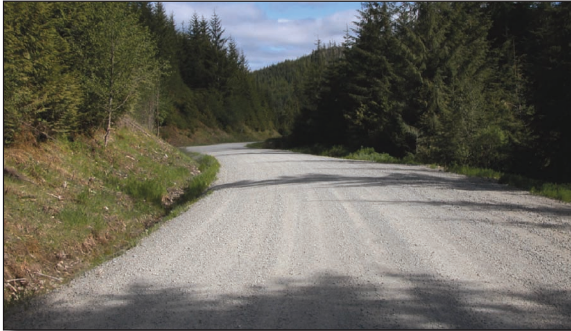
Figure 6—Maintenance level 4 double-lane road with a gravel surface and gravel shoulders. The crown is effective for gravel-surfaced roads to facilitate drainage and maintain a fully functioning surface. This road has been properly bladed to provide a moderate degree of user comfort and convenience. Ditches are kept clean to facilitate drainage. The road is free of litter and the maintenance of the roadside vegetation provides adequate sight distance. Curves and other hazards should be marked with warning signs if advised by a documented engineering judgment or engineering study. Heavy traffic may require dust abatement to maintain standard.
