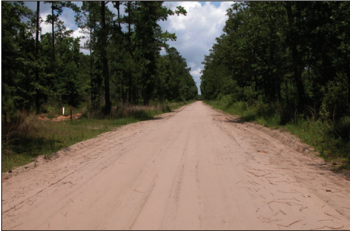
Figure 16—Maintenance level 3 double-lane road with a native surface and shoulders. Maintain road surface to provide adequate drainage. The road is free of litter. Maintenance of roadside vegetation provides adequate sight distance. Surface roughness and rutting is acceptable if maintained for travel by a prudent driver in a standard passenger car. User comfort and convenience are not considered priorities.
