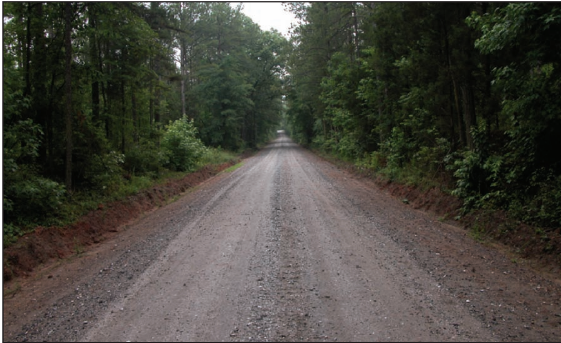
Figure 11—Maintenance level 4 single-lane road with a gravel surface and gravel shoulders with ditches. The ditches have been cleaned out to facilitate proper drainage. Maintain proper crown, repair potholes, and remove washboarding to facilitate drainage and to maintain a moderate degree of user comfort and convenience at moderate travel speeds. Replace surfacing to the depth required for blade maintenance and to prevent wear of the base course. The roadside vegetation is becoming overgrown and should be maintained to provide adequate sight distance.
