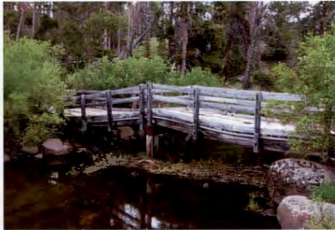
Example of a failing trail bridge, Beaverhead-Deerlodge National Forest, Montana.
